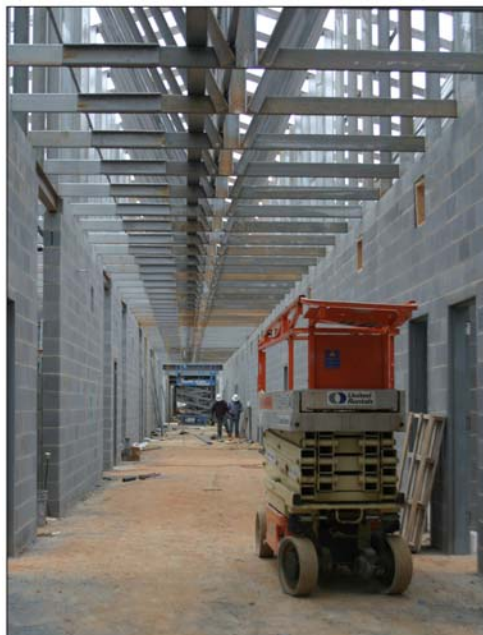
This is a view of a hallway from the eighth grade classroom wing at Middle School #4. The building is based on a prototype design first used for Springfield Middle School. The building is located on Banks Road and will be accessible from the southern leg of the Fort Mill bypass (Springfield Parkway).
